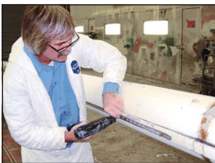
The spars are moved into the paint shop and fastener removal begins. Master technician, Earl Hadcock, starts by removing the few movable screws using a battery powered screwdriver but finishes the process using a grinder to buzz the heads off seized machine screws.
