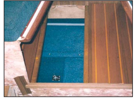
Teak and holly floor is laid over the original carpeted space below the vee berth and a hatch cutout for bilge pump access. Note bulkhead prepped for veneer.
