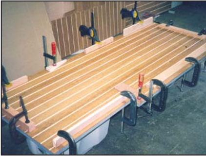
Gluing and clamping of teak and holly floor to marine plywood subfloor.
