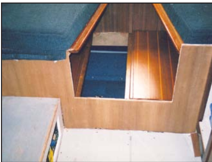
(top) Contact cement is applied to mating surfaces of the bulkhead and the teak veneer. (bottom) Teak veneer glued to bulkhead.
