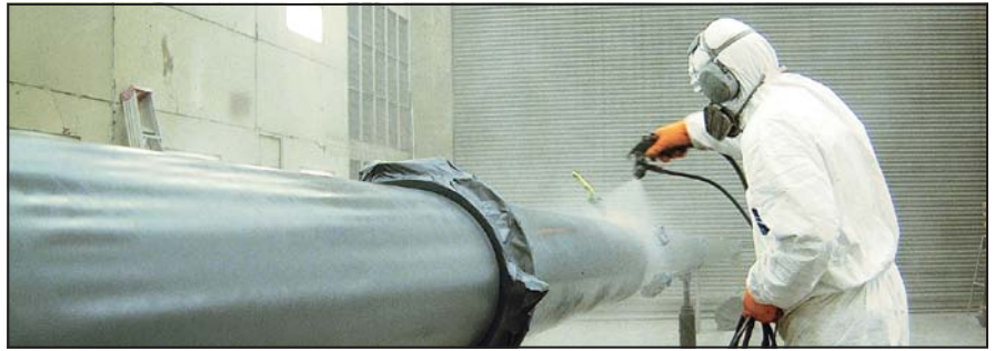
Two coats of epoxy primer (medium build) are applied by pressure-pot spray gun. Note the loss of paint as overspray.
