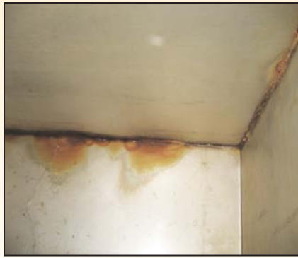
Corrosion along the weld lines created pinhole leaks in this freshwater tank.
